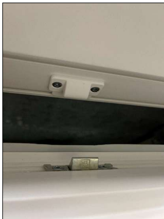
Photo 1: Restrictors in top frame and sash (DTI, 2022)
