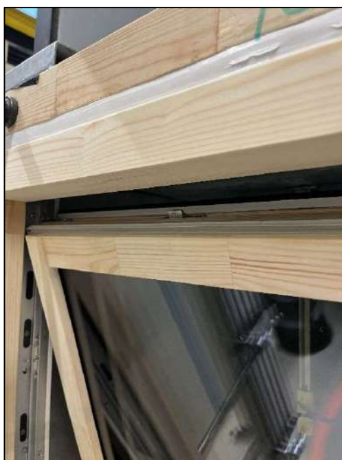
Photo 1: Restrictors in top frame and sash (DTI, 2022)
